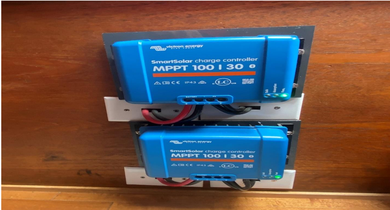
Solar Charge Battery Control
