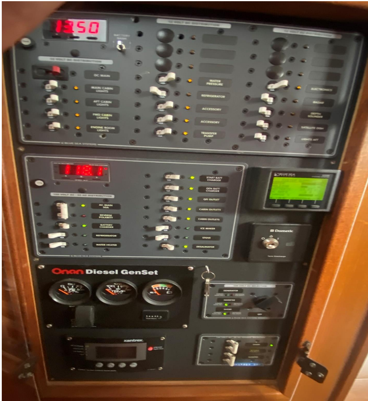
New (2017) - AC / DC Blue Sea Array Panel – Onan Diesel GenSet / 120V-AC Selection + Source Selector / Xantrex Battery Modes / Blue Sea System- Water-Holding-Battery-DC Amps- Charge % (sighted)
