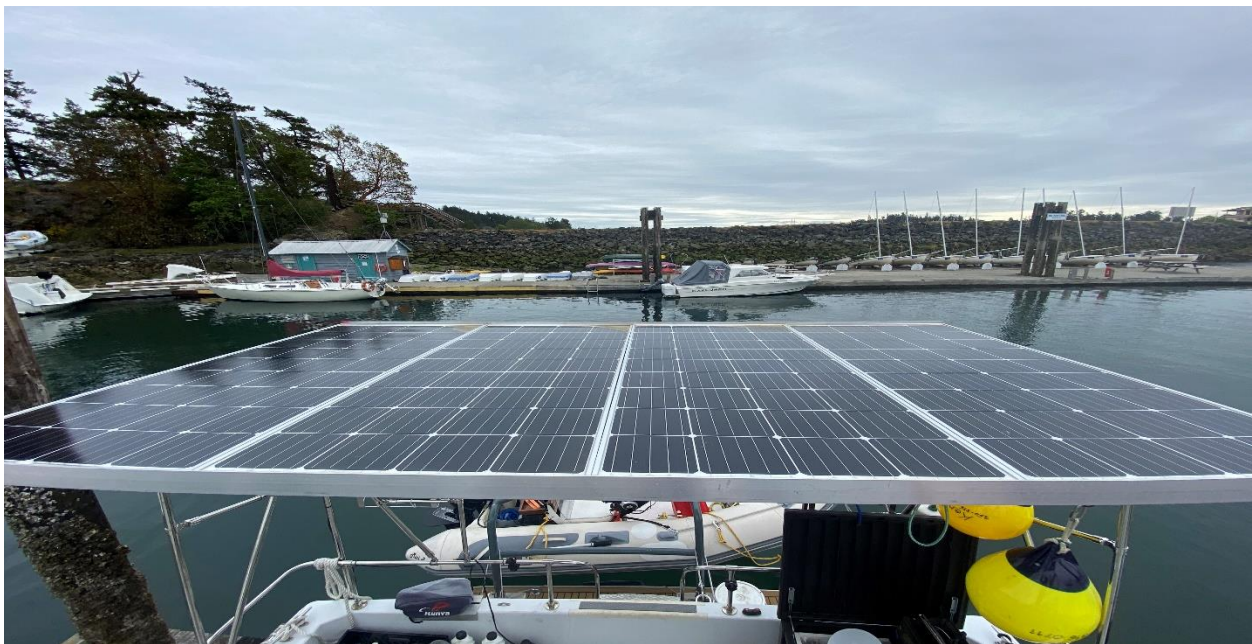
Solar Panel Array - 3000W
