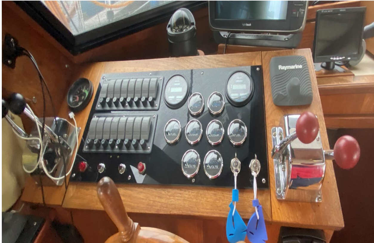
DC Helm Array / Throttles – Shifts / DC Breakers
